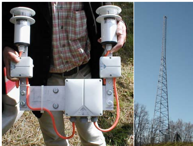
To the left a set of redundant LED flares as they are now installed on every mast, like on the one to the right.
